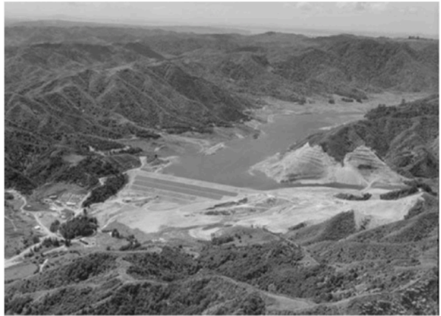
Mangatawhiri Dam under construction, Hunua Ranges, Auckland Region, 12 February 1965. Whites Aviation Ltd: Photographs. Ref: WA-63449-F. Alexander Turnbull Library, Wellington, New Zealand. http://natlib.govt.nz/records/22347942 .
